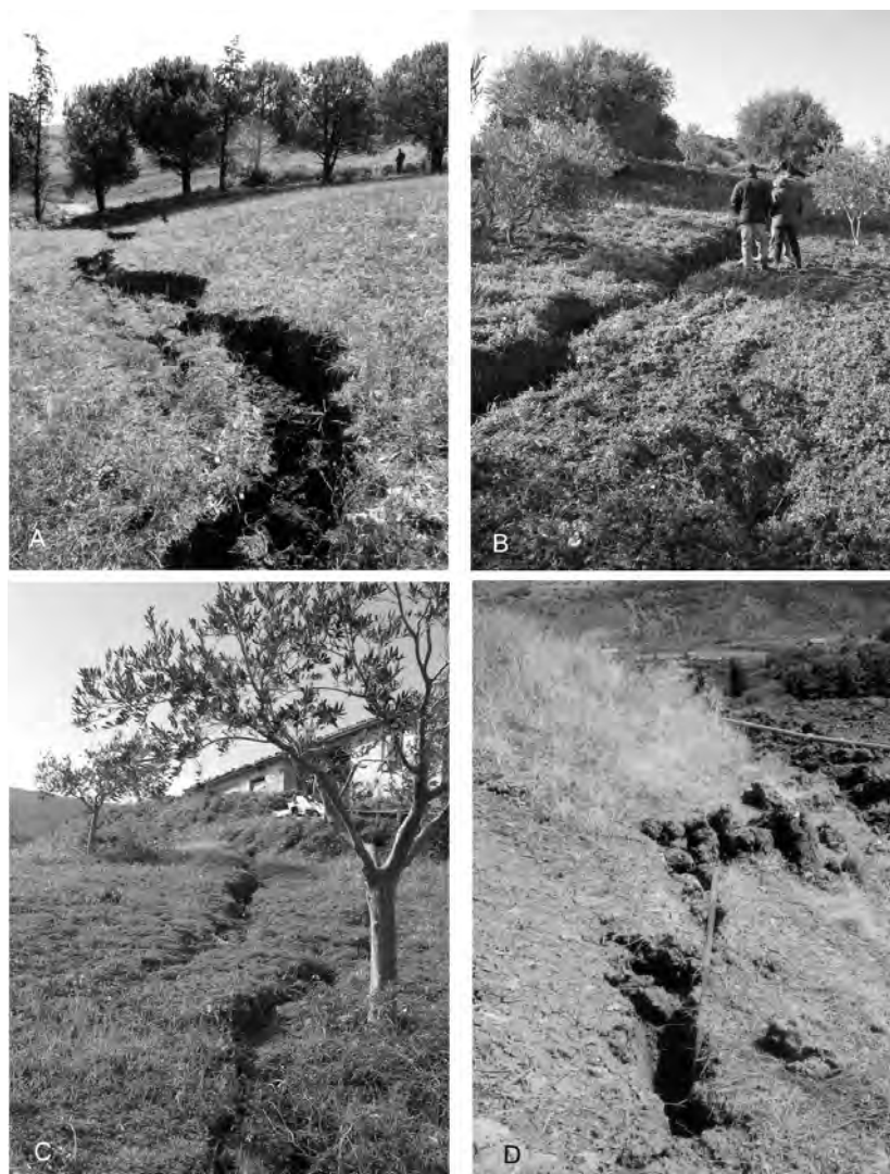
Fig. 3 - Ground cracks within the landslide mass some days after the 6, September, 2002 reactivation (by the CERI team group): a, b) normal cracks in the active zone of the landslide; c) strike-slip crack in the neutral zone of the landslide; d) inverse crack in the passive zone of the landslide.
