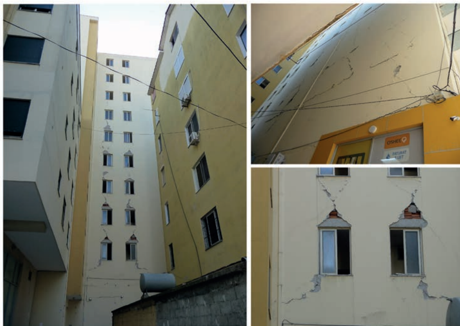
Fig. 2 - Images of damaged masonry infills of one reinforced concrete building (Ruga Pavaresia) after the 21 September 2019 earthquake.
