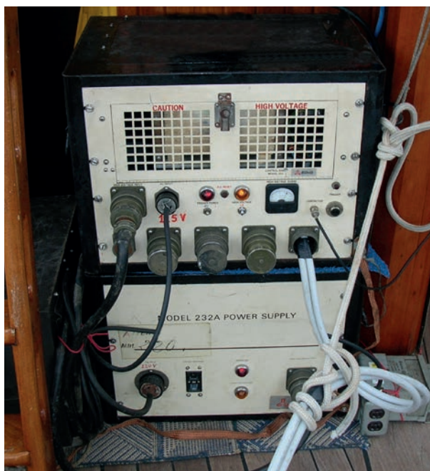
Fig. 5 - Power system EG&G, mod. 231-232.
