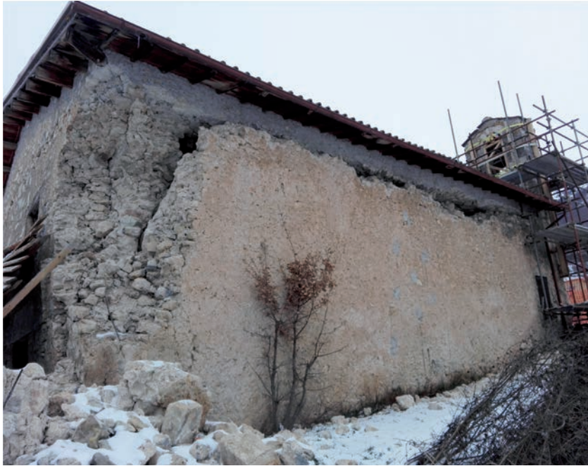
Fig. 7 - Church of Santa Giuliana, in San Pellegrino, Norcia (Perugia province, central Italy). The heavy beam supporting the roof is an intervention that introduced significant differences of stiffness or mass increase in the upper part of the building.
