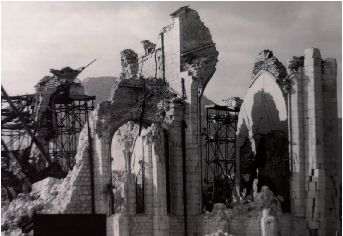
Fig. 5 - Progression of damage (modified from Doglioni et al. , 1994): the cathedral of Venzone a few days after the earthquake of 6 May 1976 (top) and after the events of September 1976 (bottom).
