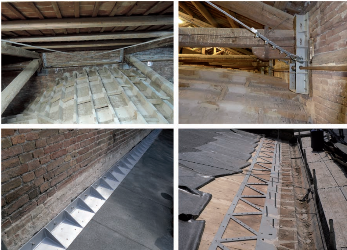
Fig. 8 - Example of problem-specific interventions based on Code of Practice criteria. Tailored solutions defined for the roof of the church of Beata Vergine Maria in Ostiglia (Mantua province) damaged by the 2012 earthquake in Emilia (northern Italy).
