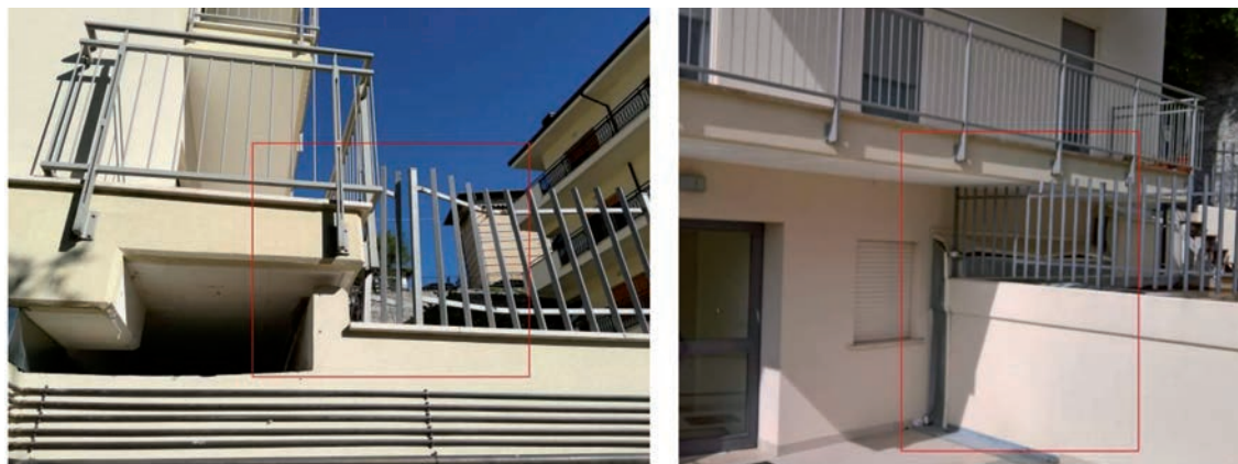
Fig. 8 - Damages of the interface elements installed between the isolated structure and the fixed one (metal casings, fence, etc.).
