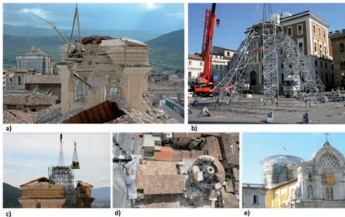
Fig. 2 - Short-term countermeasures for securing the dome of Anime Sante cathedral in L'Aquila after the 2009 Abruzzo earthquake, realized by CNVVF: a) damage situation of the dome; b) preparation of the “octopus” in a safe place; c) mounting operations by crane; d) in-place “octopus”; e) completed work.
