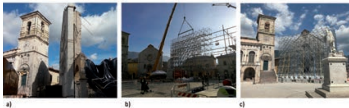
Fig. 4 - Short-term countermeasures for securing the façade of the San Benedetto basilica in Norcia (Perugia province) after the 2016 central Italy earthquake: a) the damage situation after the 30 October 2016 main-shock; b) positioning by crane of the scaffold structure built in safety place; c) completed securing works.
