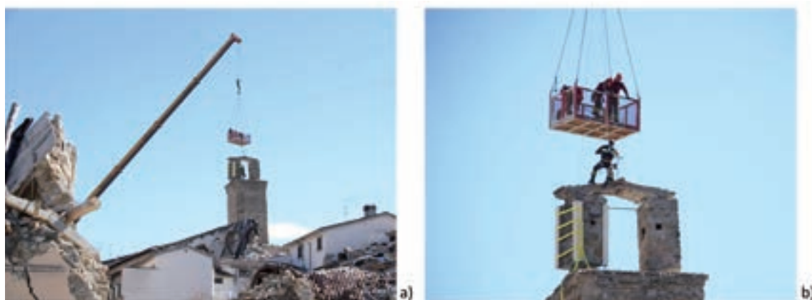
Fig. 9 – Controlled dismantling of the remaining parts of the bell tower of the Civic Tower of Amatrice (Rieti province), still standing after the main-shock of October 30, 2016: a) view of the intervention work from a distance; b) close up view.
