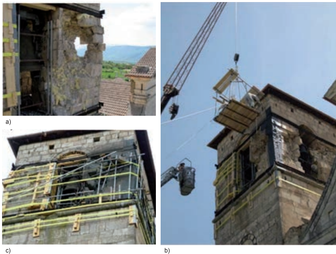
Fig. 3 - Short-term countermeasures for securing the bell tower of the San Felice Martire church of Poggio Picenze (L'Aquila province) realized by CNVVF after the 2009 Abruzzo earthquake: a) damage situation of the bell tower; b) application of carbon-fibers for reinforcing the damage pillar; c) completed intervention.
