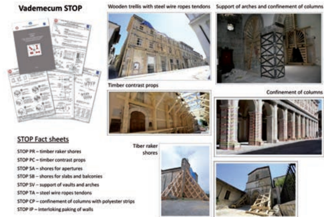
Fig. 1 - Vademecum STOP. Shoring template and operating procedures for securing buildings damaged by earthquake. On the left: fact sheets for different standardized solutions. On the right: examples of STOP solutions.
