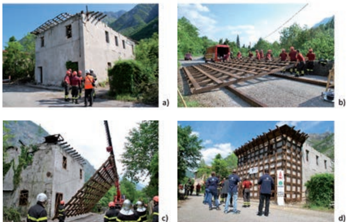
Fig. 7 – Construction stages of the experimental solution (trellis laterally anchored): a) initial situation of the old kindergarten with roadside facing wall; b) preparation of the trellis in a safe area; c) positioning the trellis with a crane; d) completed work with lateral anchoring steel wire tendons.
