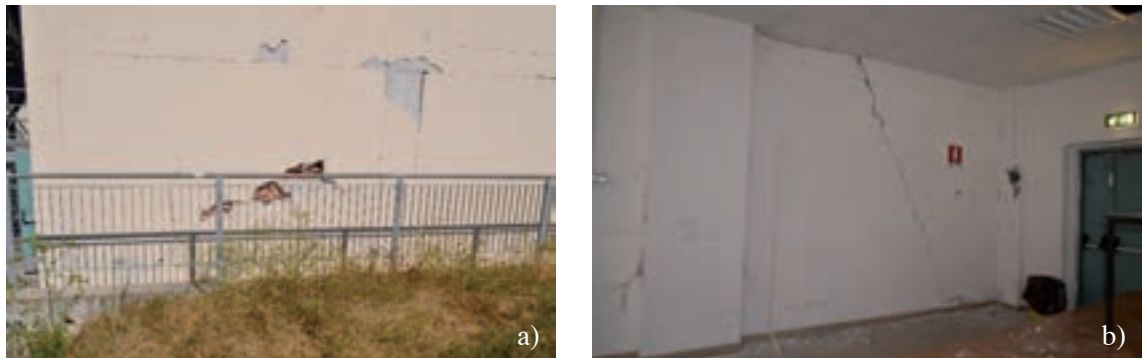
Fig. 13 - R. Battaglia RC frame building: a) poor connection between structural and non-structural elements; b) diagonal and some sub-horizontal cracks in non-structural masonry infills.
