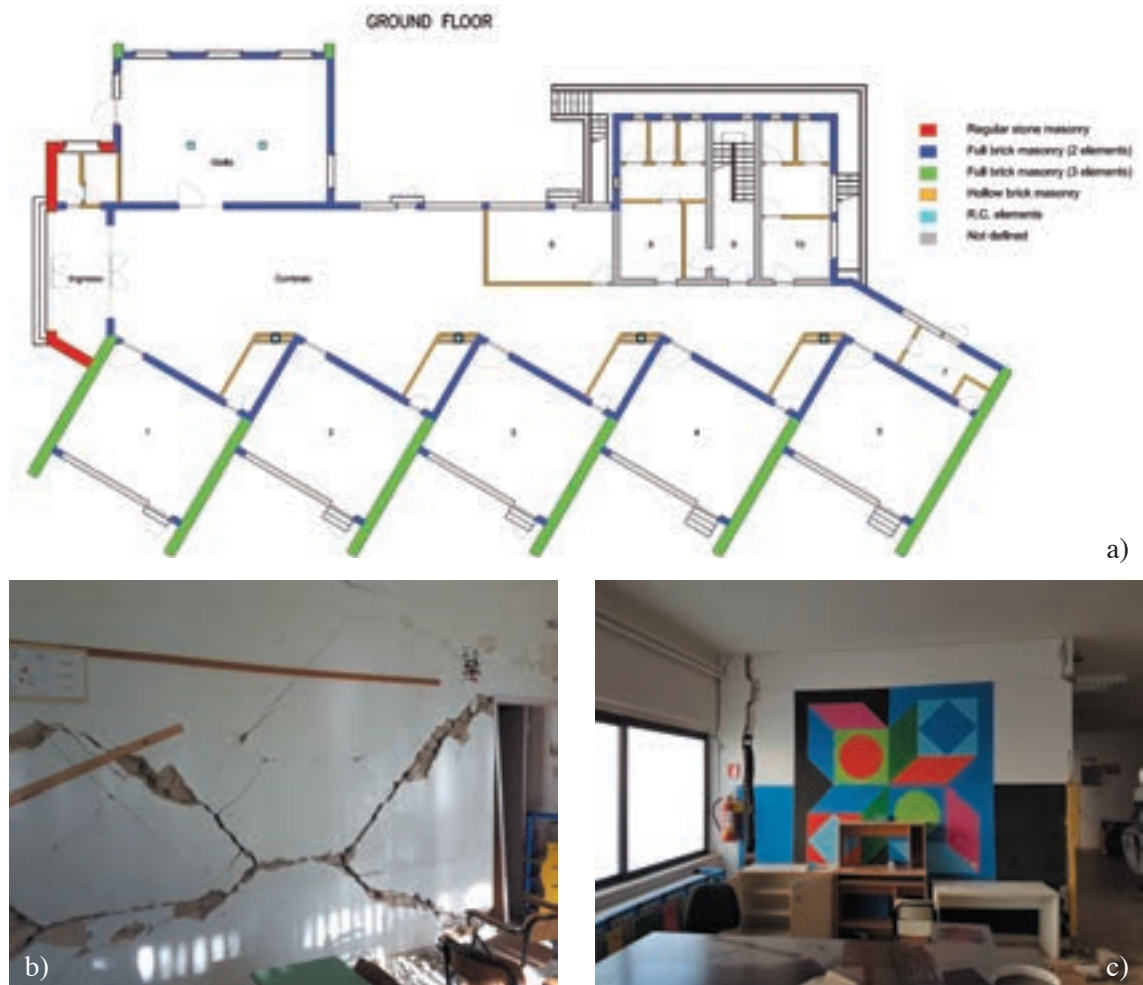
Fig. 16 - Mons. Paoletti elementary school building: a) ground floor plan with indication of structural elements; b) diagonal and c) sub-vertical cracks in non-structural masonry infills.
