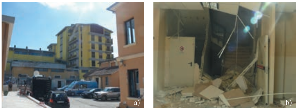
Fig. 14 - The Hotel Management school of Amatrice: a) external view of the building; b) collapse in the hall and damage of RC stairs.
