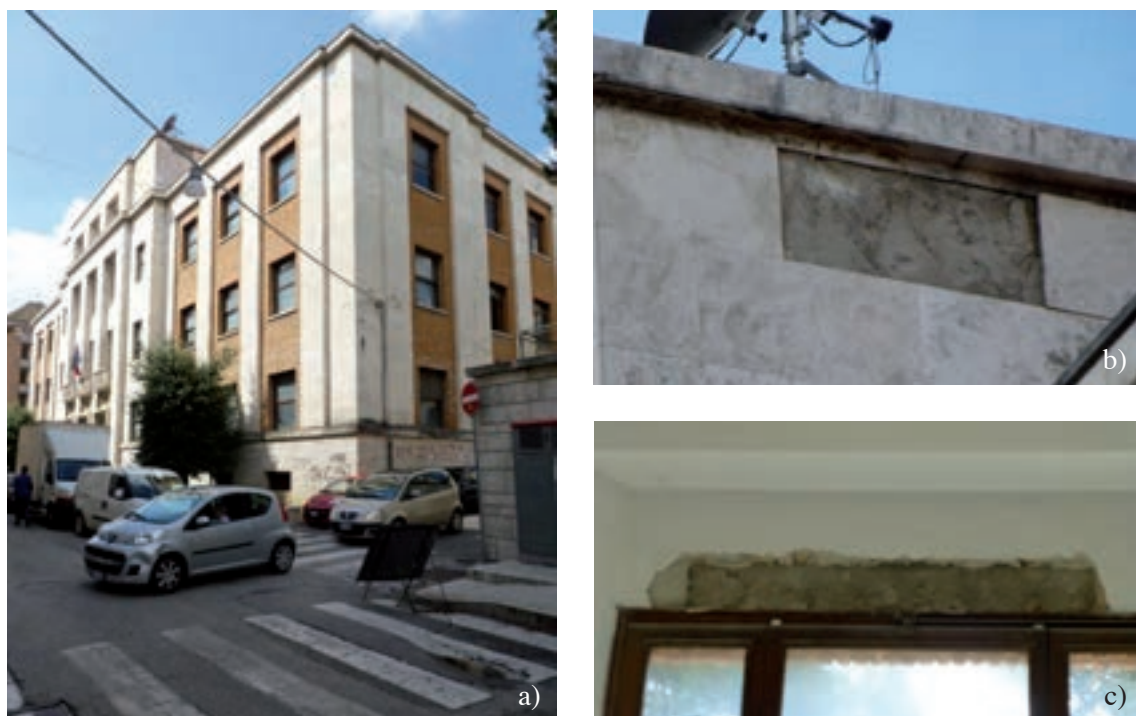
Fig. 11 - G. Milli high school building: a) external view of the complex; b) detachment of a travertine plate; c) detail of the collapsed plaster cover of the window lintel.
