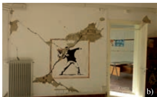
Fig. 20 - The elementary school of Pievebovigiana: a) ground floor plan; b) shear cracks in an inner wall of the east pavilion.
