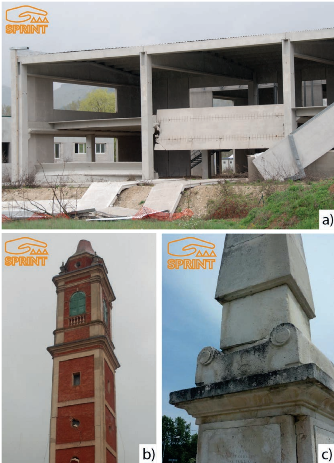
Fig. 10 - a) Precast building in L'Aquila (Monticchio, Italy). The damage could be ascribed to joint presence of vertical and horizontal ground motion in a friction based-system. b) Bell towers showing a clear cut at the cusp: bell tower of the church of S. Martino in Buonacompria – Cento (FE, Italy) (date of the photo: May 21, 2012). c) Rotation of a symmetrical obelisk (Mirandola, Emilia, Italy 2012).
