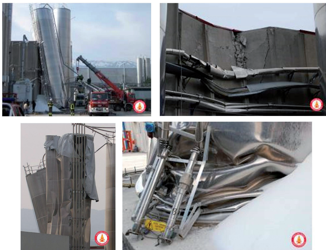
Fig. 1 - L'Aquila earthquake: damage to, and caused by, silos at VIBAC facility in the Bazzano industrial area, 7 km south far from L'Aquila town.
