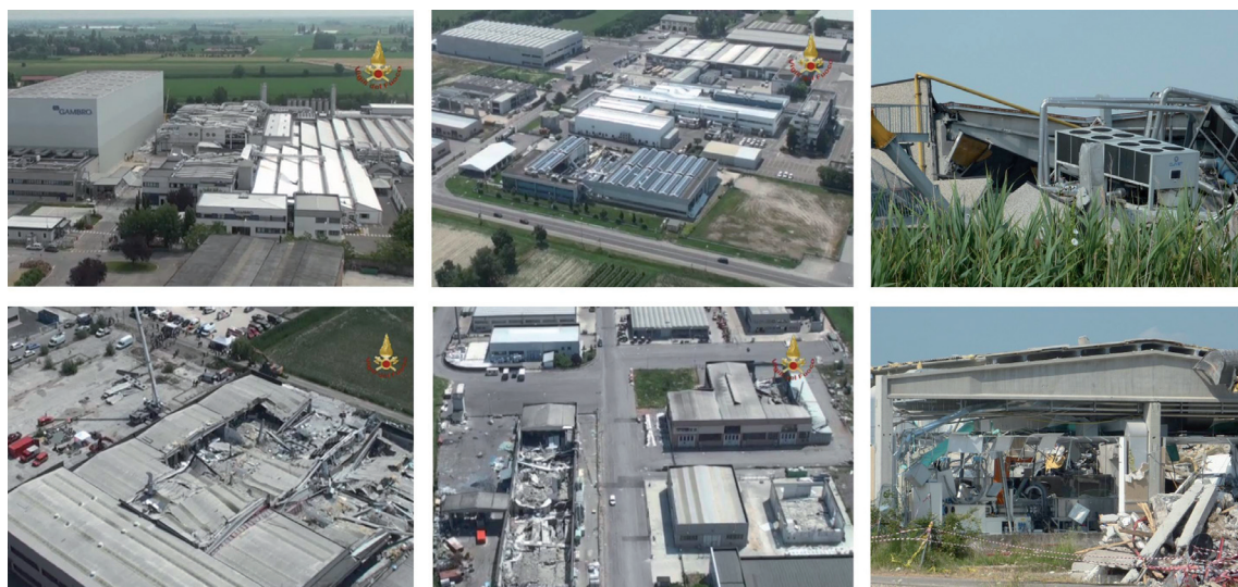
Fig. 2 - Emilia earthquake: heavy damage to industrial buildings in the epicentral area. General collapse of roof of precast system structures destroyed the internal facilities.
