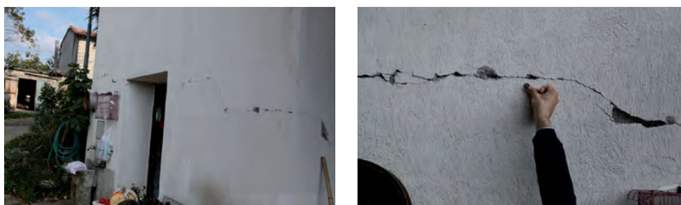
Fig. 10 - View of the most damaged building in Rotonda after the October 26, 2012 earthquake.
