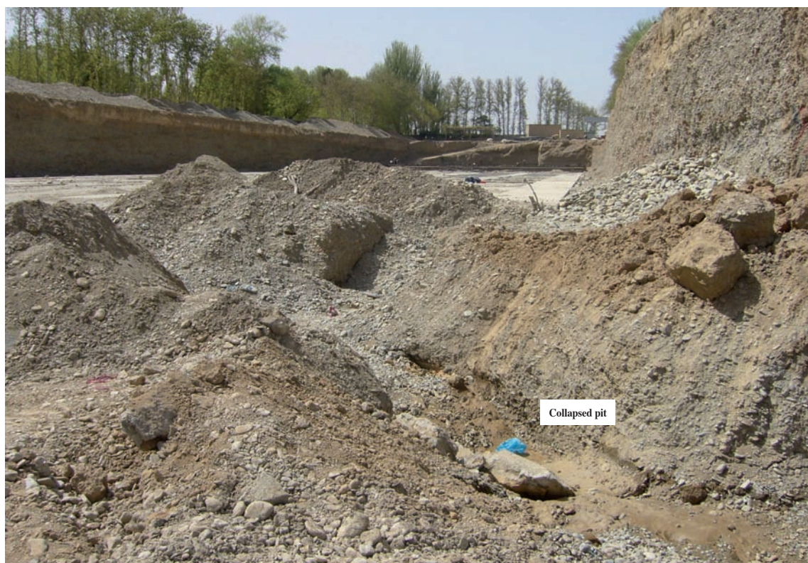
Fig. 1 - Foundation and collapsed pit.
