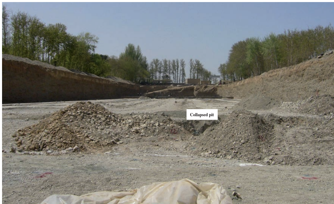
Fig. 2 - Foundation and collapsed pit.
