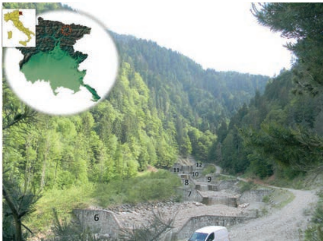
Fig. 1 - View of the investigation area from the northern side. The check dams are numbered according to the reference scheme adopted in the text.
