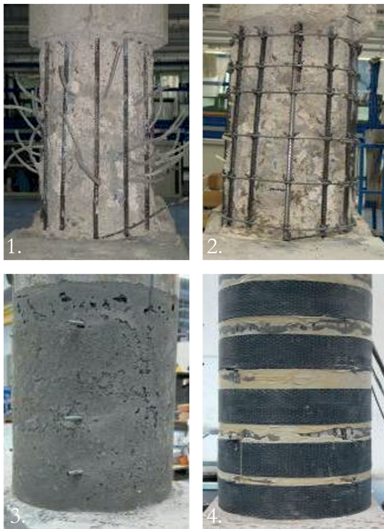
Fig. 7 - Experimental samples of CFRP application onto a concrete column, in the following order: 1) removal of damaged concrete and epoxy resin injections; 2) replacement of the bars; 3) restoration of the concrete surface; 4) application of transverse and longitudinal CFRP jacketing.
