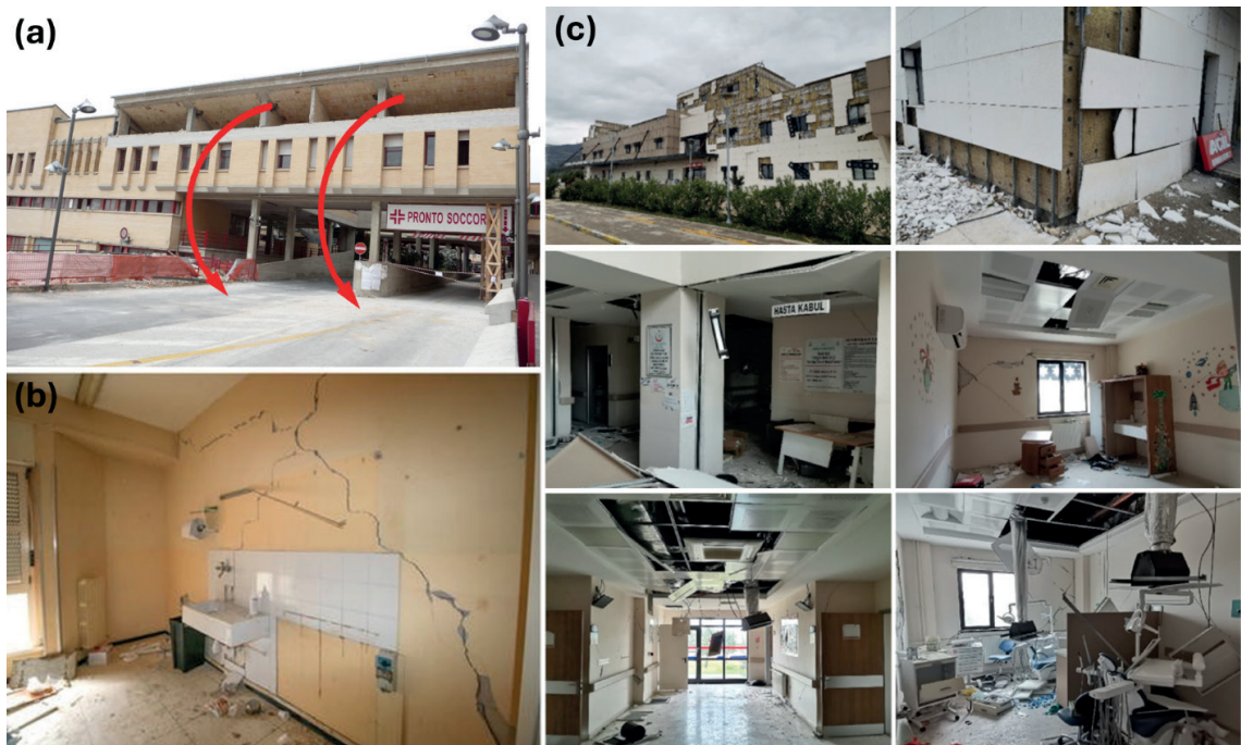
Fig. 1 - Non-structural seismic damage observed in hospitals: a) full collapse of masonry infill panels above the entrance portico, San Salvatore Hospital following the 2009 L'Aquila earthquake (Price et al. , 2012); b) severe cracks in internal masonry partitions, the hospital in Amandola following the 2016-2017 central Italy seismic sequence (Santarsiero et al. , 2019); and c) critical damage to various non-structural elements including architectural systems and building contents, Nurdaği State Hospital following the 2023 Turkey earthquake sequence (Qu et al. , 2023).
