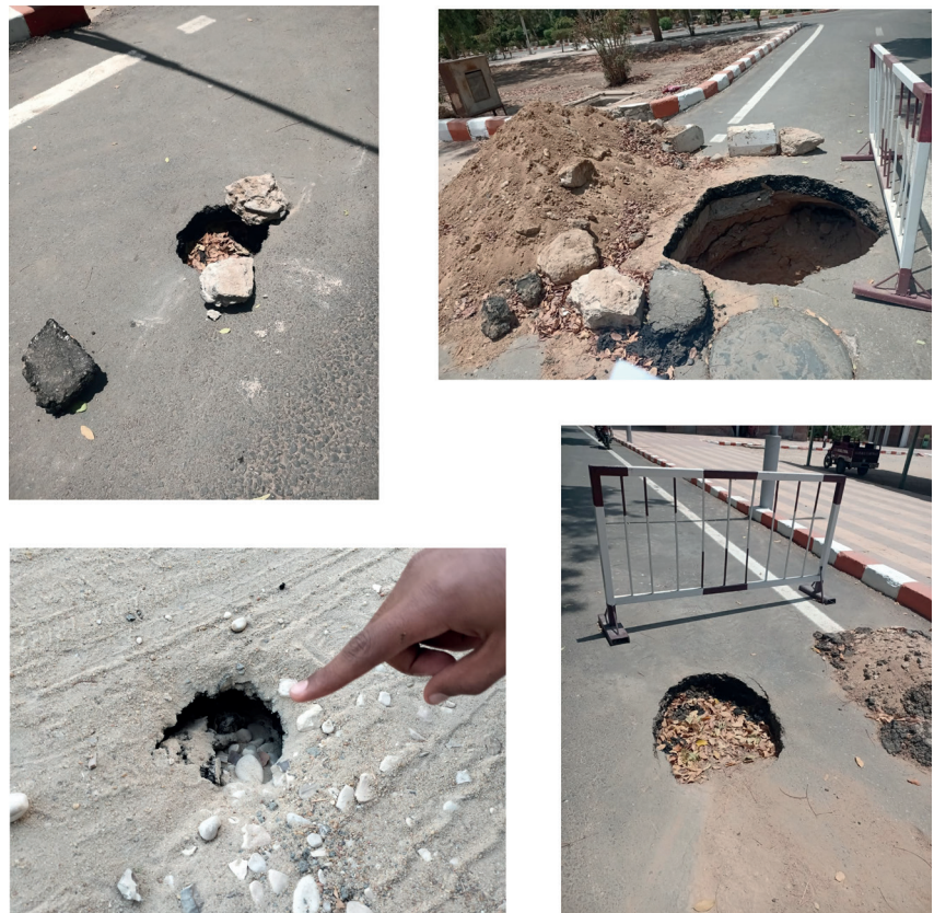
Fig. 3 - Images show the pits opened in the asphalt roads, as a result of collapses in the subsoil.
