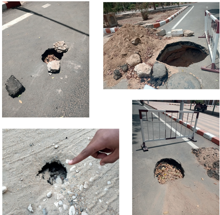
Fig. 3 - Images show the pits opened in the asphalt roads, as a result of collapses in the subsoil.
