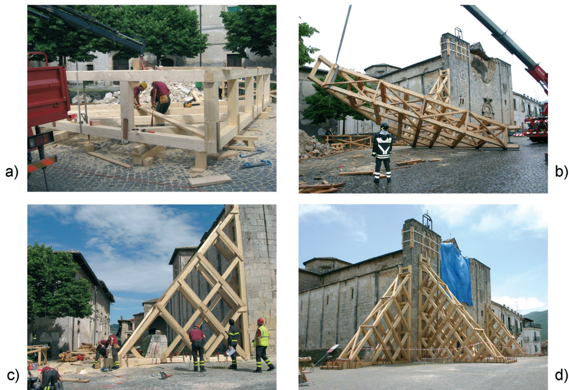
Fig. 5 - Shoring of the church of Sant'Eusanio Martyr in Sant'Eusanio Forconese (AQ). A standard solution provided in the vademecum STOP has been adopted: a) assemblage of the structure on the ground in a safe place; b) lifting of the structure by crane; c) positioning of the structure and anchorage at the base; d) provisional work completed.
