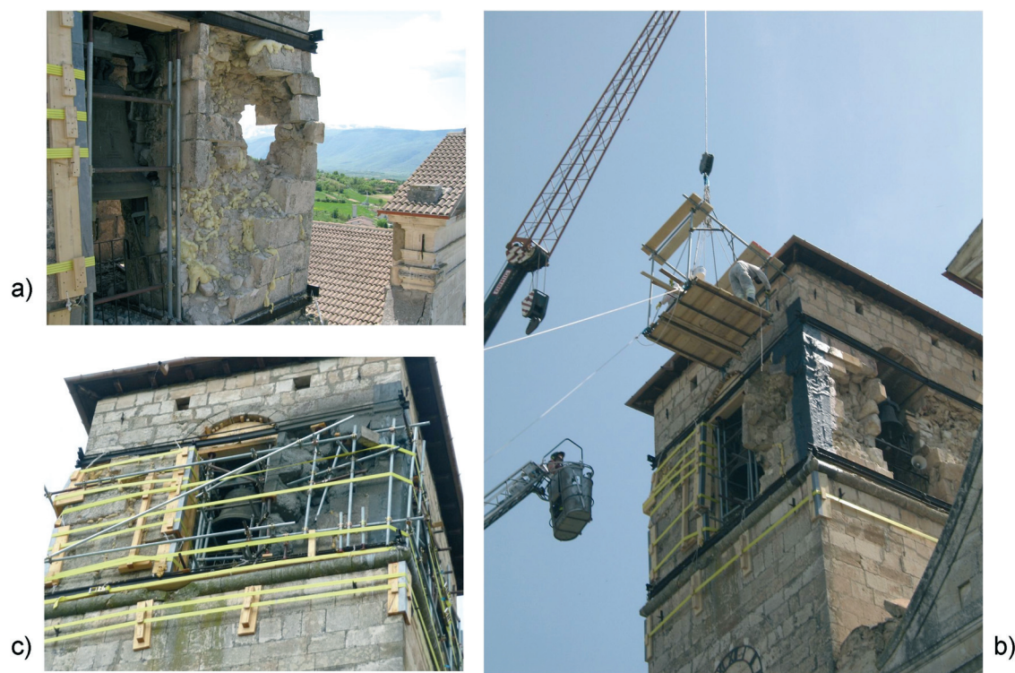
Fig. 6 - Intervention to secure the belfry of the steeple of the church of San Felice Martyr in Poggio Picenze (AQ) by using carbon fibre: a) the precariousness of stability generated by damage to the bell tower with the possibility of collapse onto the church; b) application of carbon fibres by using techniques from the staff share in CNVVF-SAF; c) securing of the belfry completed.
