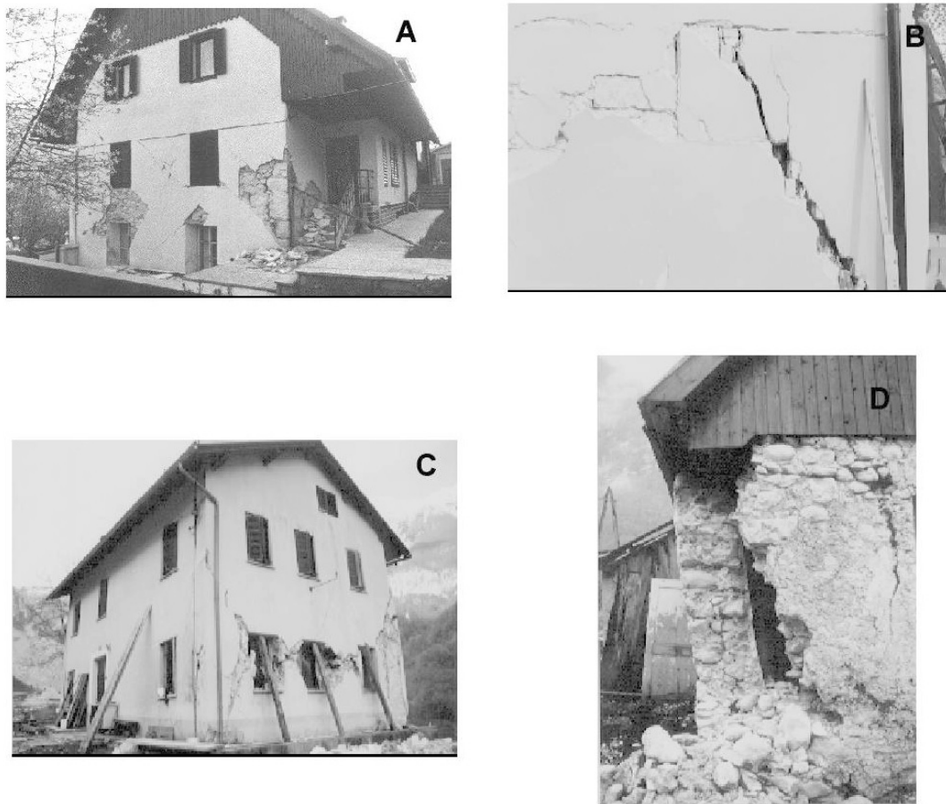
Fig. 9 – Examples of structural damage on buildings in the epicentre zone: Drežniske Ravne (A), Mala Vas (B), Javorca (C) and the Lepena valley (D).
