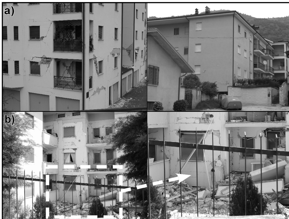
Fig. 9 - a) Casantessa, examples of damage of grade 3 in buildings with vulnerability classes C and D; b) Pettino, via Dante Alighieri, damage of grade 4-5 in buildings with 'theoretical' vulnerability class D (to be declassified to C).
