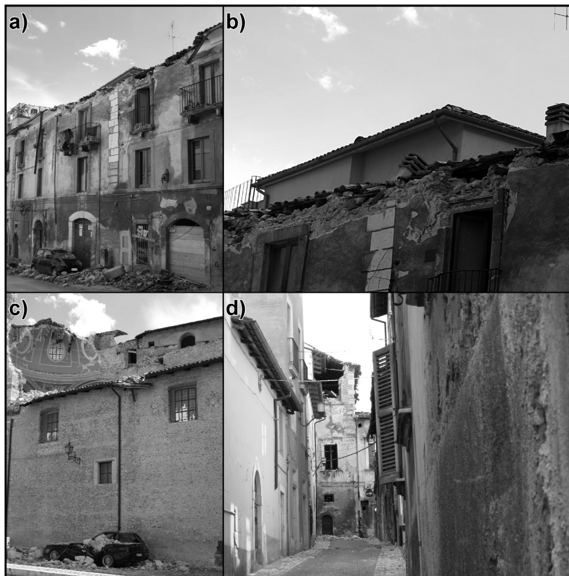
Fig. 7 - L'Aquila, historical centre, examples of damaged buildings with different vulnerability: a) ancient edifice with unsatisfactory maintenance; b) detail, the height of the building has recently been raised by one storey; c) church of St. Maria Paganica; d) restored and well-maintained houses coexist with abandoned ones, sharing lateral load-bearing walls.
